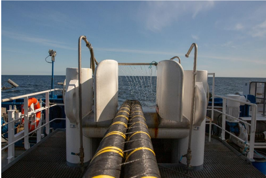
Meter by meter, the NordLink submarine cables are lowered into the sea. ©TenneT
